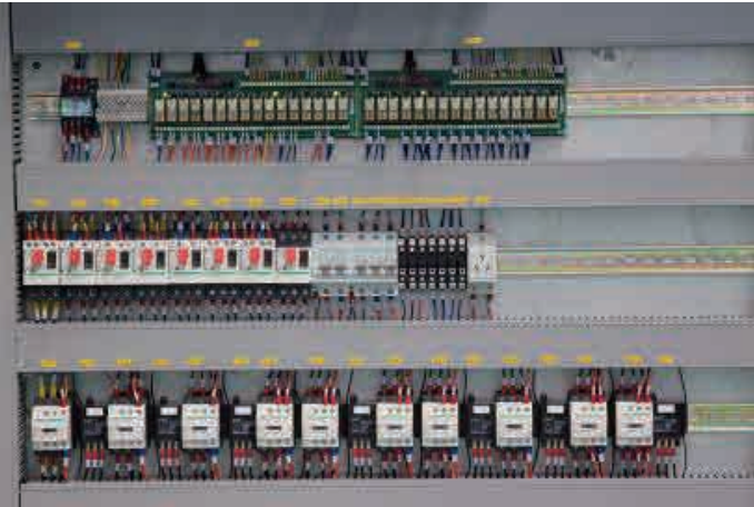
• The electrical cabinet is arranged neatly and orderly, and the cable and wire serial numbers are marked, which is convenient for maintenance and fault finding and shortens the trouble shooting time.
